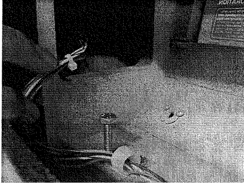
Inside Top Box: Left Side
