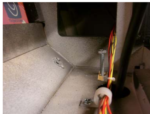
Inside Top Box: Right Side
